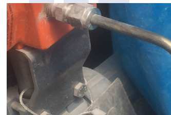
Tungum installed with twin ferrule stainless steel compression fittings, more than 12 years in service with no corrosion issues.
